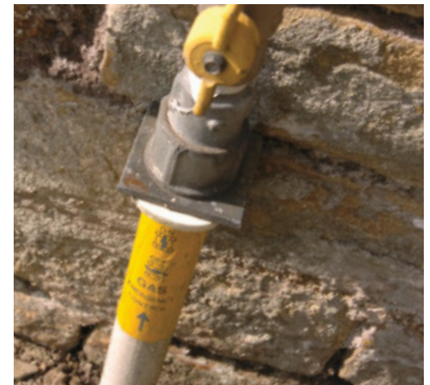
Pipework protected from below ground to emergency control
