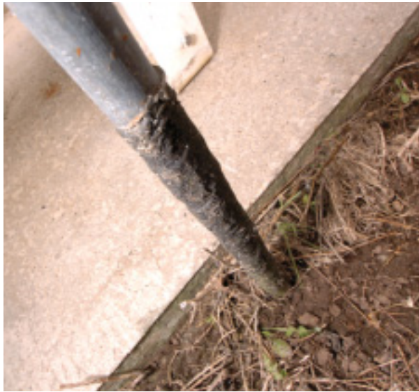
Metallic pipework protected as it enters the ground
